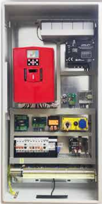
MR Control Panel
